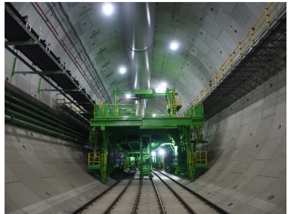
Tunnel Construction Site at Tomei JCT (Source: Tokyo Outer Ring Road Project Website)
