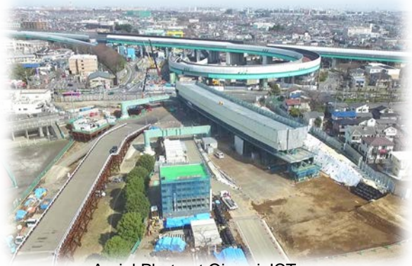
Aerial Photo at Oizumi JCT (Source: Tokyo Outer Ring Road Project Website)
