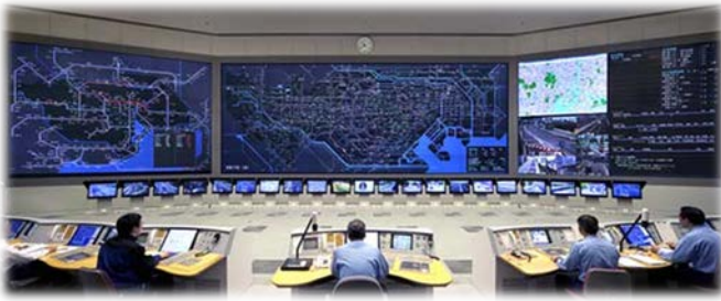
Traffic Control Center (Source: Tokyo Metropolitan Police Department Website)
